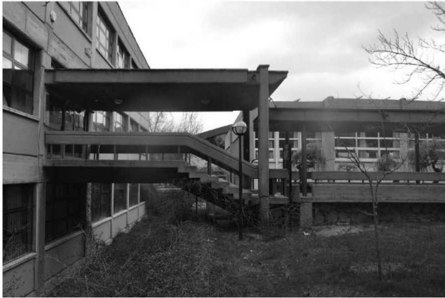
Figure 150. Electric and Electronics department A block entrance and arcades, photograph by the author, 2022
